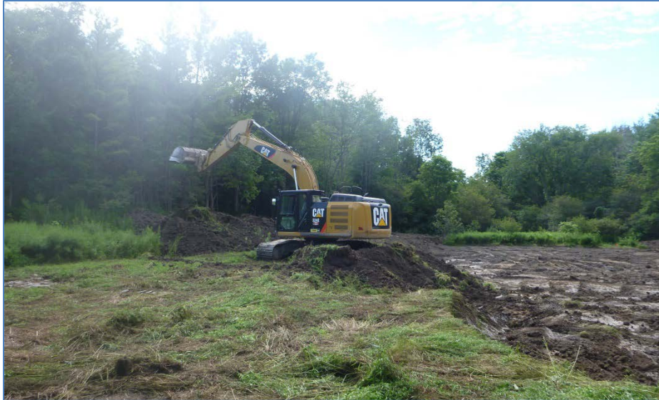
Wetland excavation on a landowner's property in the Headwaters of the Sydenham River.
